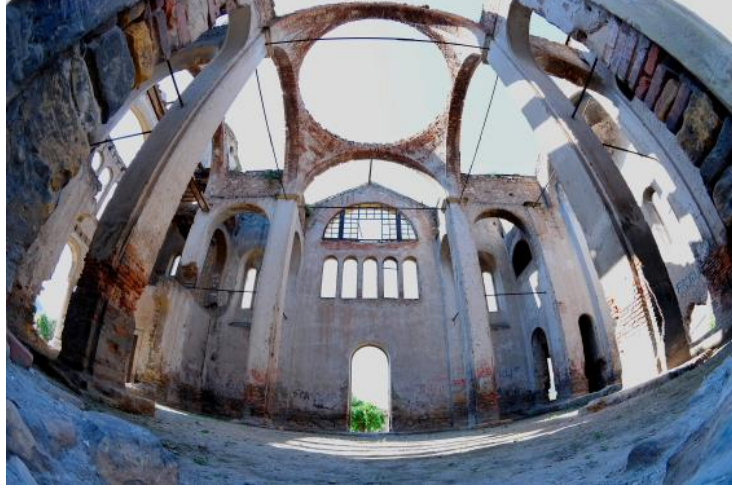
Figure 7. Deformations in masonry pillar ( https://www.osmaneli.bel.tr/hagios-georgios-kilisesi )
